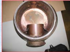
Filter Outlet Section
