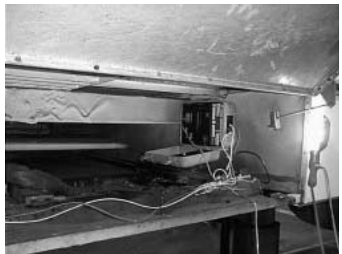
Figure 6: Data logger installation
